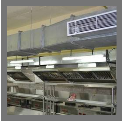
Commercial Kitchen Exhaust System
